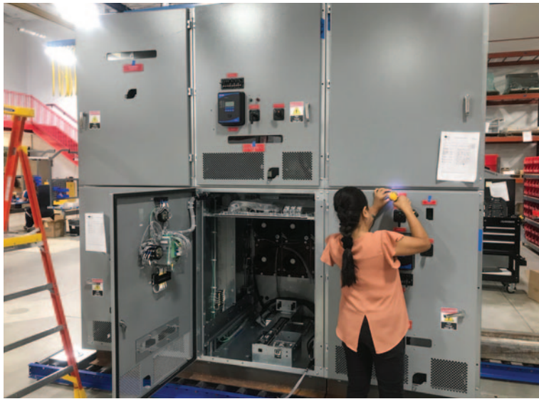
Switchgear, shown here being assembled at the new JST facility in Florida, are engineered-to-order products with a lot of variation from job to job. The firm's new sheet metal fabrication equipment allows it to excel at taking on the low-volume work.
